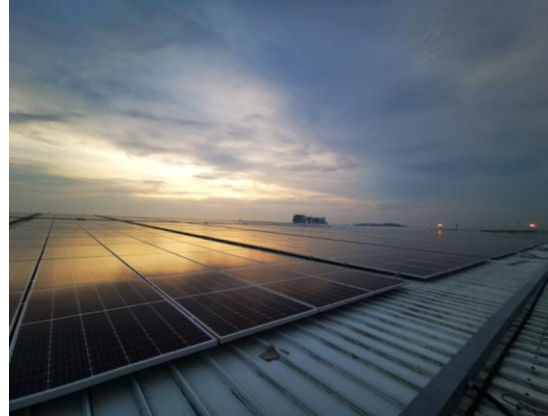
VAT Manufacturing Solar PV Installation - Side Profile
